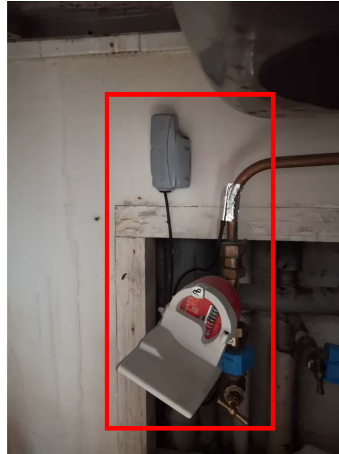
Surface temperature of DHW pipes
