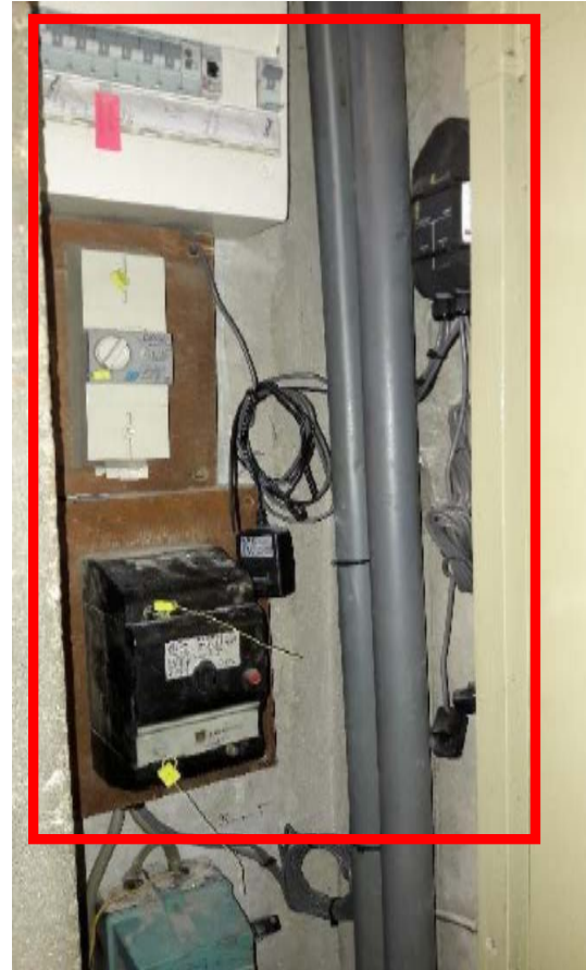
Sensor with clamp ampere meters for electric switchboard
