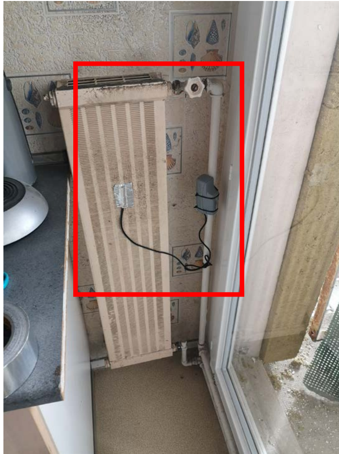
Surface temperature of heaters
