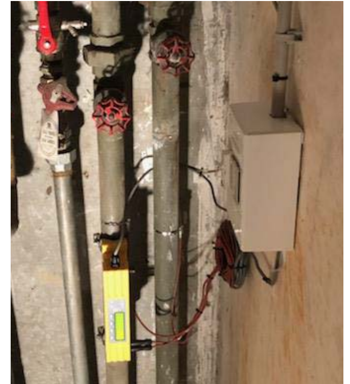
Thermal energy meter Heating/DHW energy consumption at building scale
