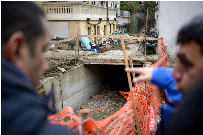
Figure 5: Photo of the culvert on top of the Ravone, near the houses we visited, after breaking during the Fall 2024 flood. Credit: Emilia Romagna region
